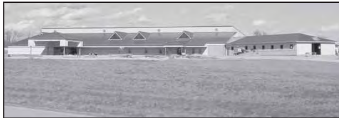
Exterior framing is finished, all roofing is complete and the facility secured with windows and doors.
